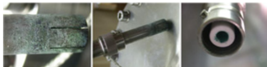
Figure 5: degradation of the outer coaxial surface
